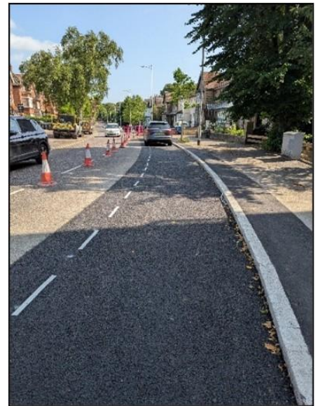
Hermon Hill hydrorock and permeable asphalt
