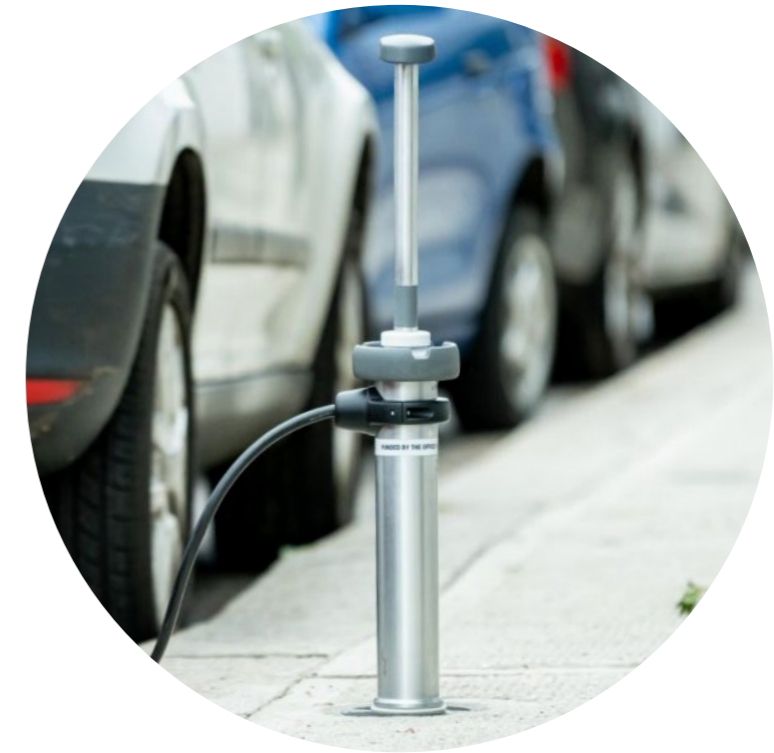
Figure 4.3 Trojan Energy chargepoint.
