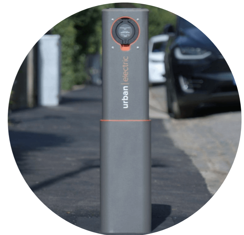
Figure 4.4 Urban Electric chargepoint.
