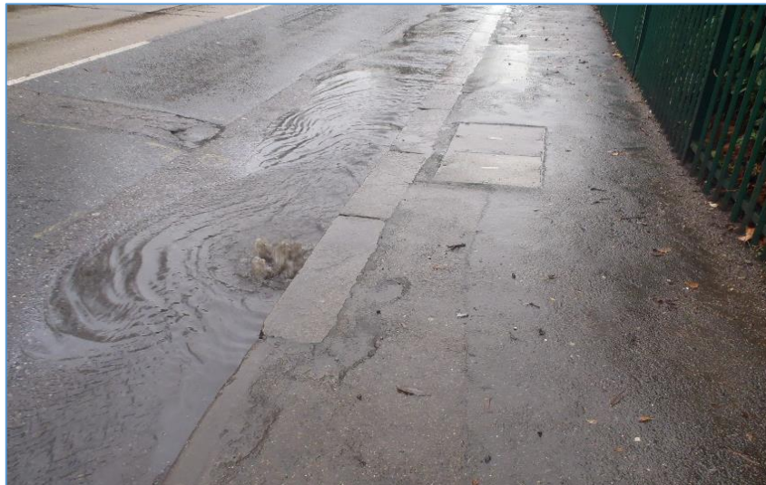
Gullies outside the school on Hainault Road. Supplied by John Martin (LBR, 2015).
