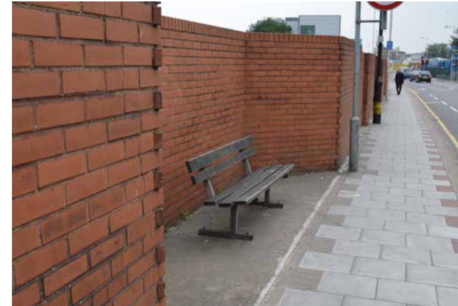
3 - The brick wall encompasses four resting places but only one has a bench.
