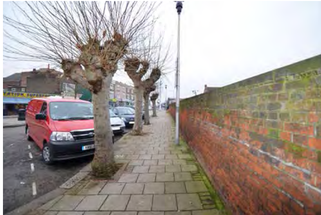
5 - A blank, brick wall forms the southern edge of the area. The wall is currently in a poor state of repair.
