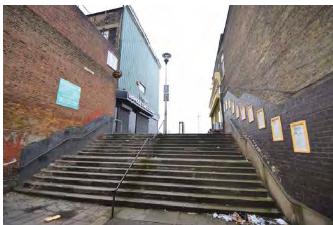
9 - The level difference and steps to Cameron Road prevents inclusivity and creates a disconnection with the activity of High Road and isolated feel to the space.
