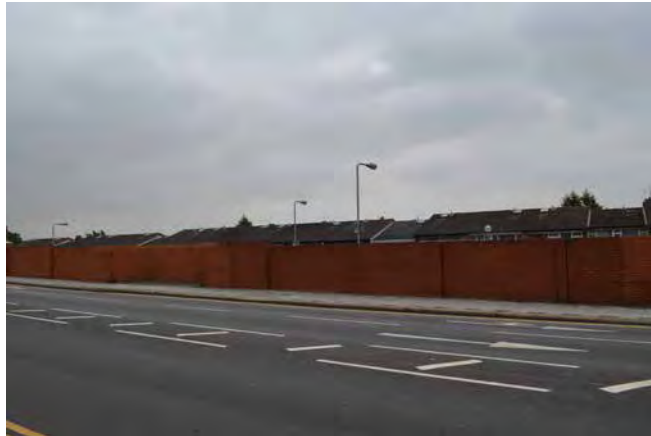
1 - Running along the southern edge of the High Road is a relatively well-maintained but blank, brick wall.
