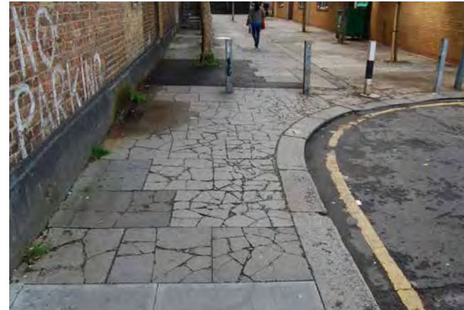
2 - Large areas of paving in poor state of repair at the northern end of Farley Drive that has been the result of turning vehicles .
