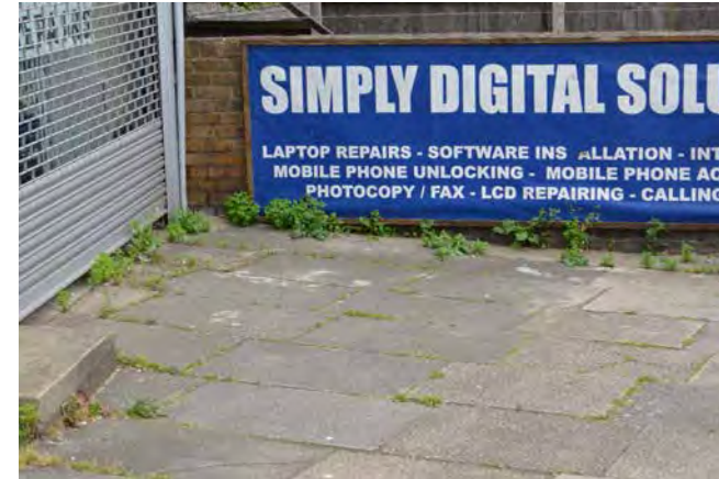
3 - Poorly maintained paving.
