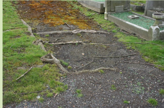
Degraded surfacing at Barkingside Cemetery
