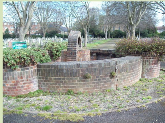
Damage to Art Deco influenced structure at Barkingside Cemetery
